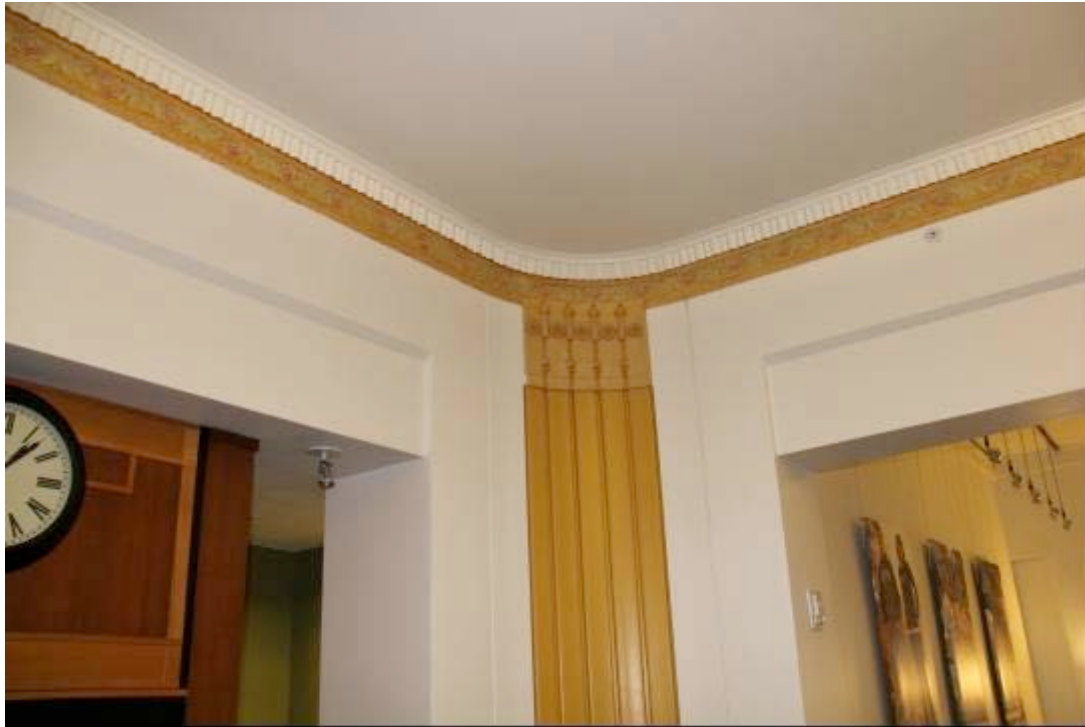
0013 Detail photo in the interior of the main entry. The ornate coving is of original construction.
