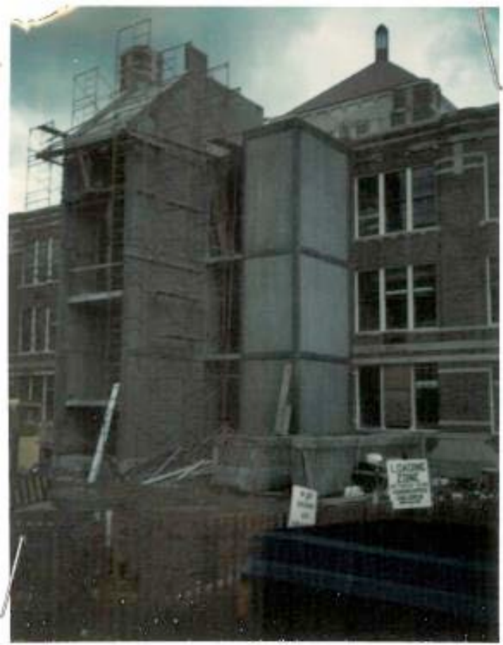
Photo looking from the northwest to the southeast of the construction of the elevator and stair tower at the back of McMullen Hall in 1971.
